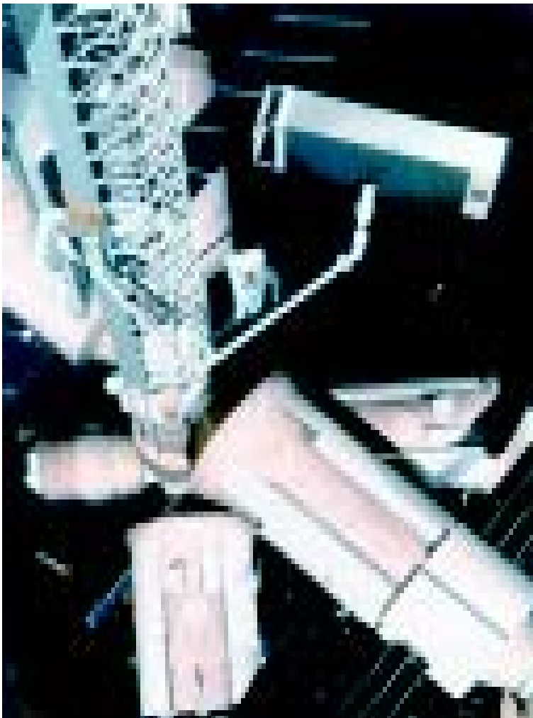
Fig. 21 Cosmonauts using the ERA to install a solar array. (source: Fokker Space)
